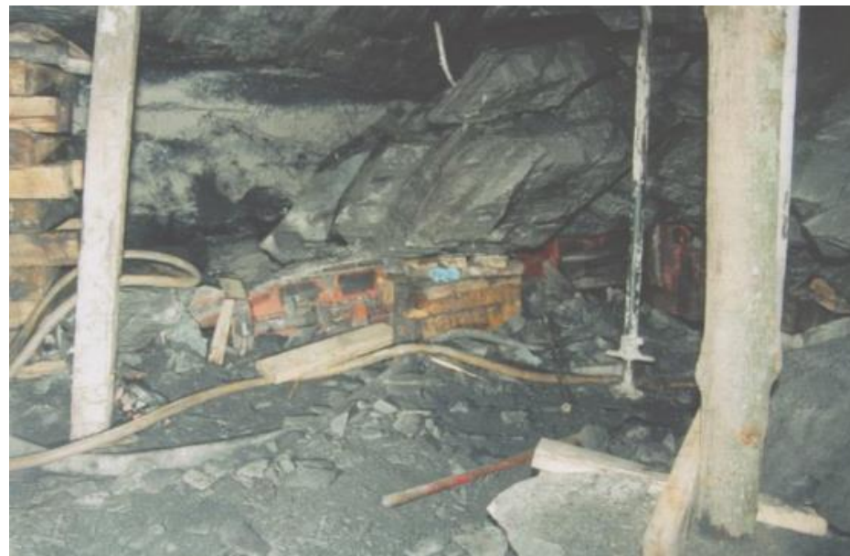
Major Roof Fall
